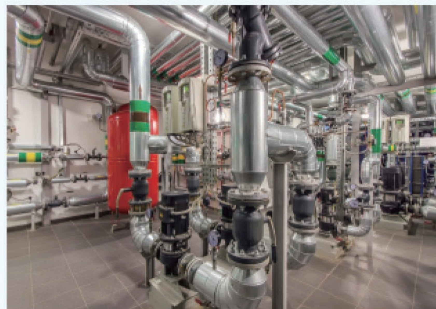
Municipal heating system
